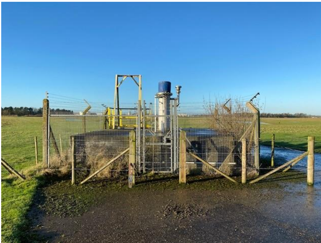
Figure 3-26: Photograph of Existing Dune Isolation Valve
